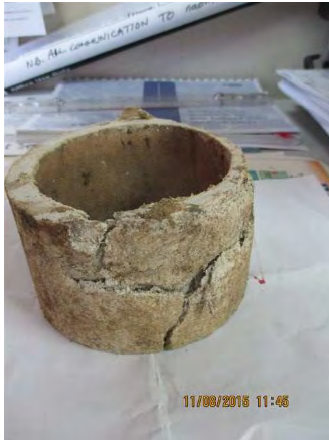
Figure 1: Collapsed water main from Mokau Indicative of reticulation condition
